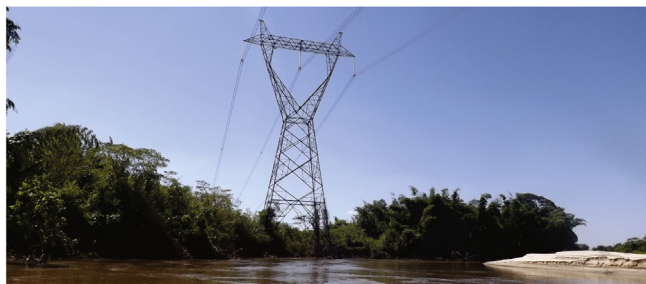
Fig. 21. Energy transmission network that needed to be relocated owing to the intense channel changes in reach 1.
