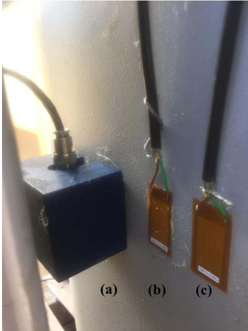
Fig. 4. Sensors installed on the transformer wall: (a) R151-AST conventional AE sensor, (b) MFC-P2 and (c) MFC-P1 sensor.
