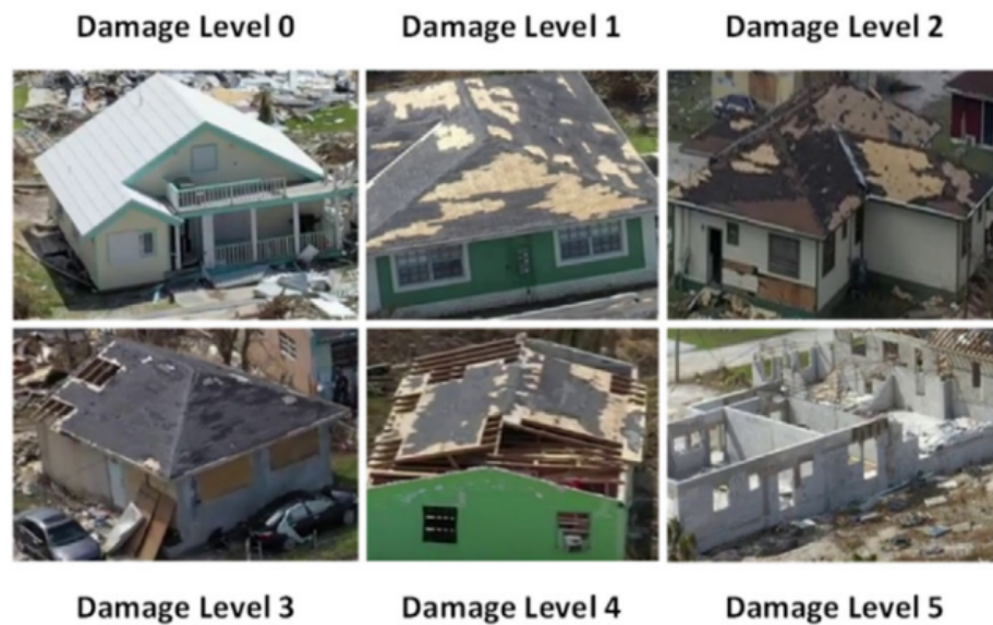
Figure 10 – Examples of constructions with different levels of damage ( CHENG; BEHZADAN; NOSHADRAVAN, 2021 ).
