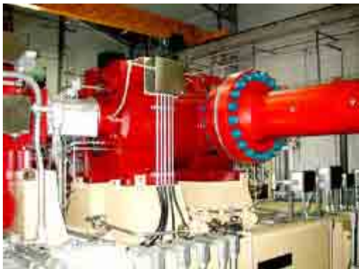
(a) Compressor de gás natural
