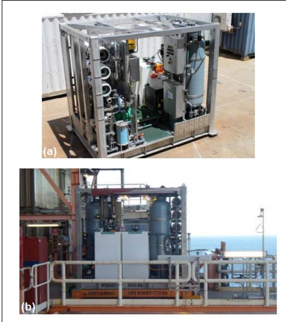
Figure 4. (a) Seawater reverse osmosis plant from MakWater (b) Installed on site.
