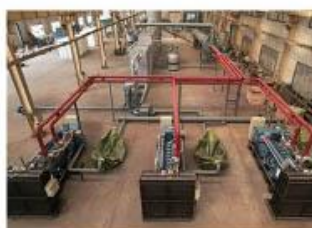
Papua New Guinea 500KW Power Plant Project
