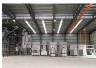
Singapore 30KW Power Plant Project
