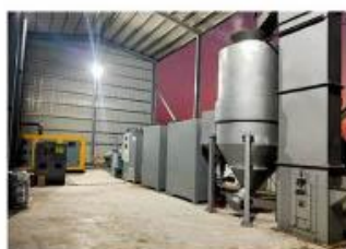
Taiwan, China 400KW Power Plant Project
