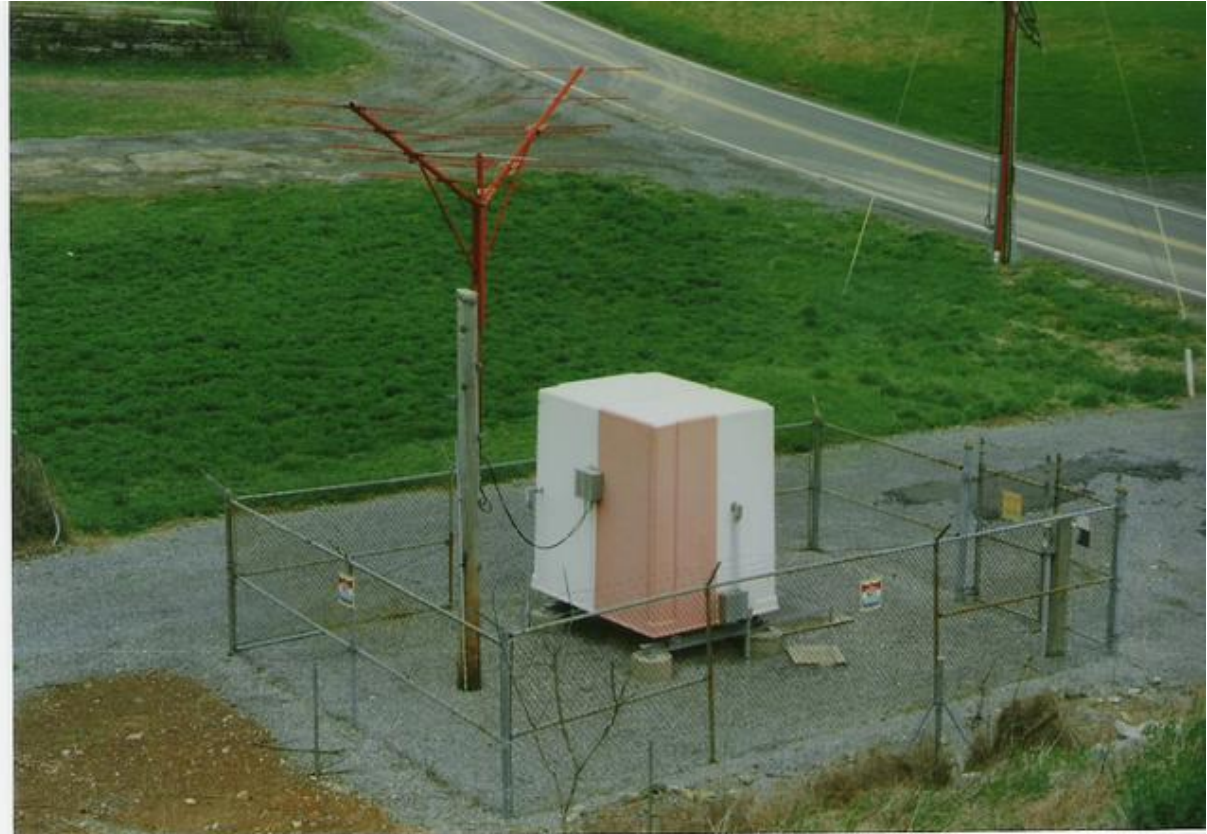
FIGURA 5.8 – Antena Marker Beacons
