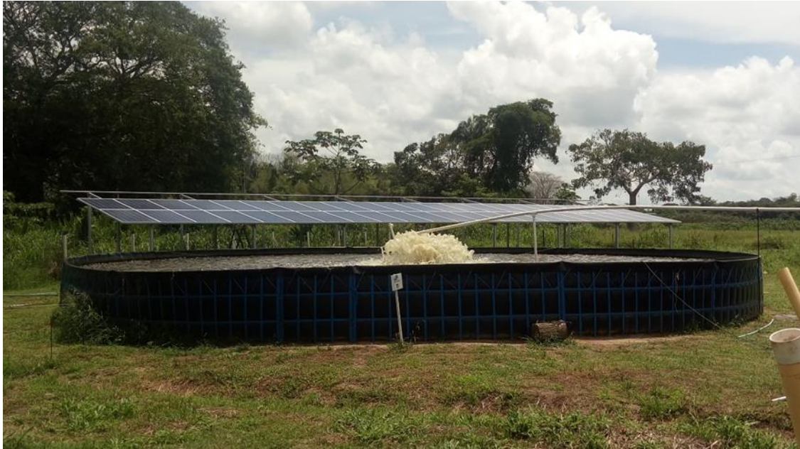
Fig. 1. Image of the production system, high-density polyethylene (HDPE) geomembrane tanks and photovoltaic system.
